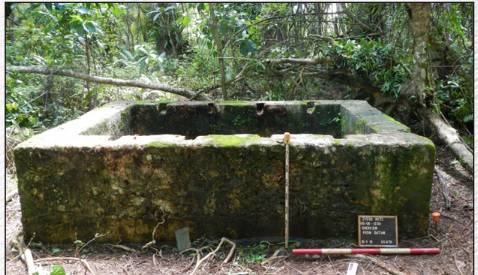
Slots along the top of the cistern probably held timbers to which a wooden lid was fastened.
